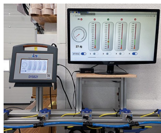
Monitoring system for cleaning nozzles
